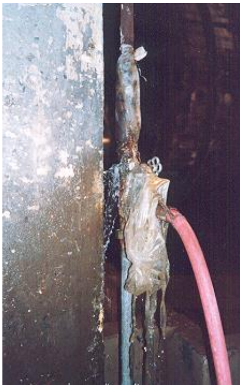
Leaking pipe connections
