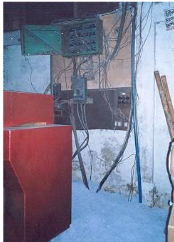
Excess use of electrical energy due to poor connections
