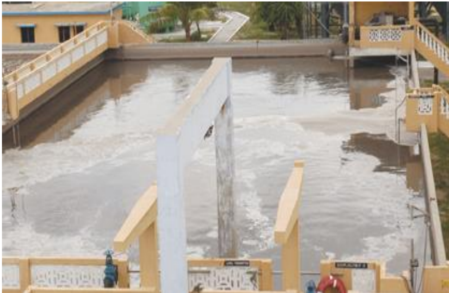
Equalization tank with jet aeration
