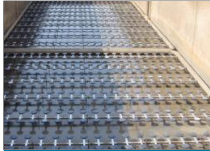
Diffusers in equalization tank
