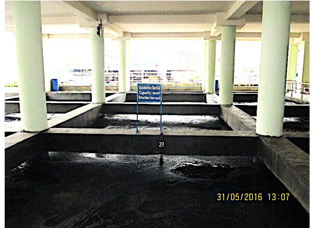
Conventional aeration tank
